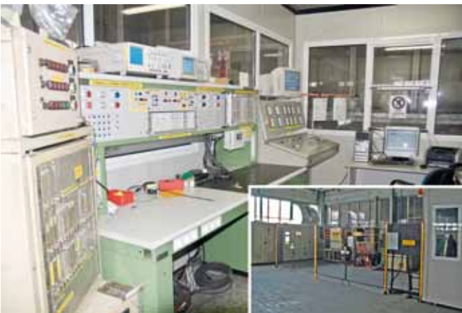
Static converter test room
